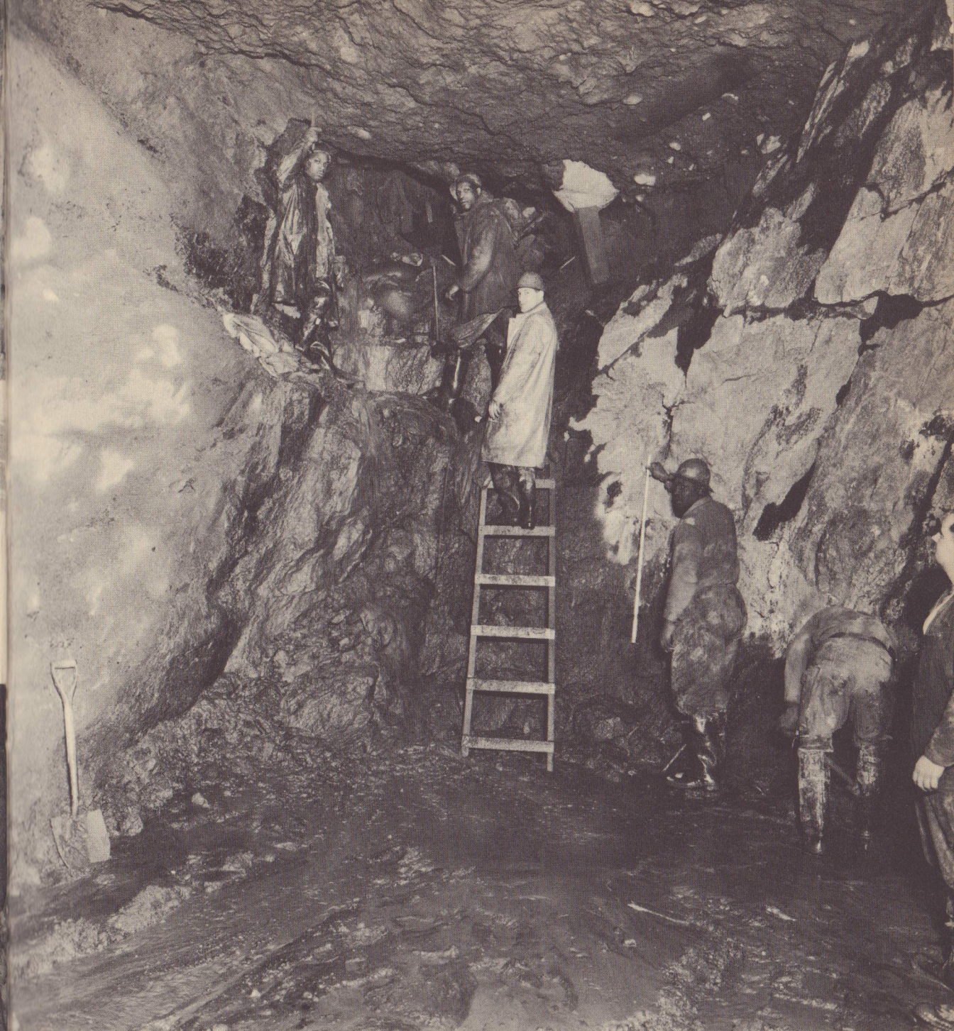
A rock tunnel has sprung a very serious leak. Note the sandbags used to hold the water and mud back. What actually happened here was that the contractor had to change his plans and change from straight rock tunneling to shield tunneling under air pressure. The test borings made at the beginning of the job did not show the break in the rock formation which caused this leak.
